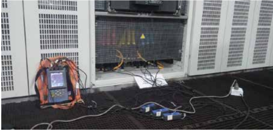
Figure 2(a) - Data Gathering Using Power Analyzer in Rolling Mill
